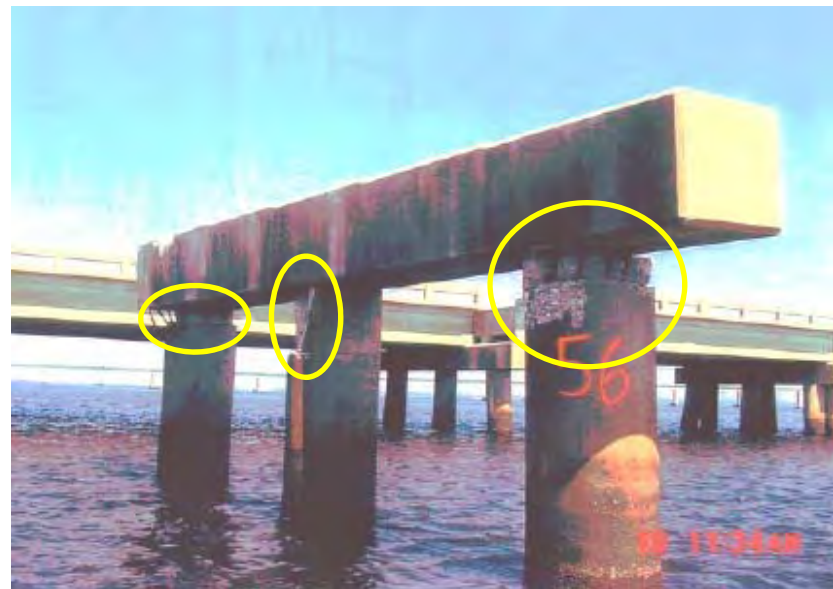
Span Dislodged Before Bent Collapsed
