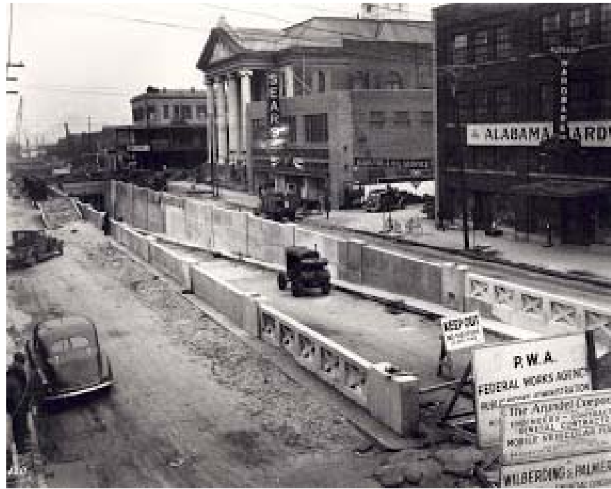
Figure 8. West end of Bankhead Tunnel under construction, ca. 1939, view to the east (The Old Mobilian 2016).
