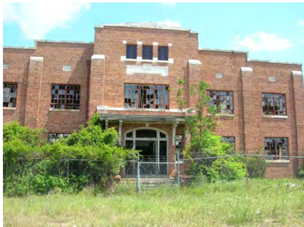
Figure 9. South façade and one of three entrances of Structure 1, main office for the ADDSCO shipyard. View to the north toward Alternates A, B, and B'.
