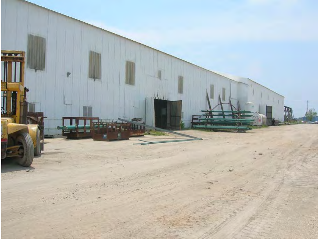
Figure 46. West side of Structure 10, former Pipe Fabrication Shop. View to the southeast.
