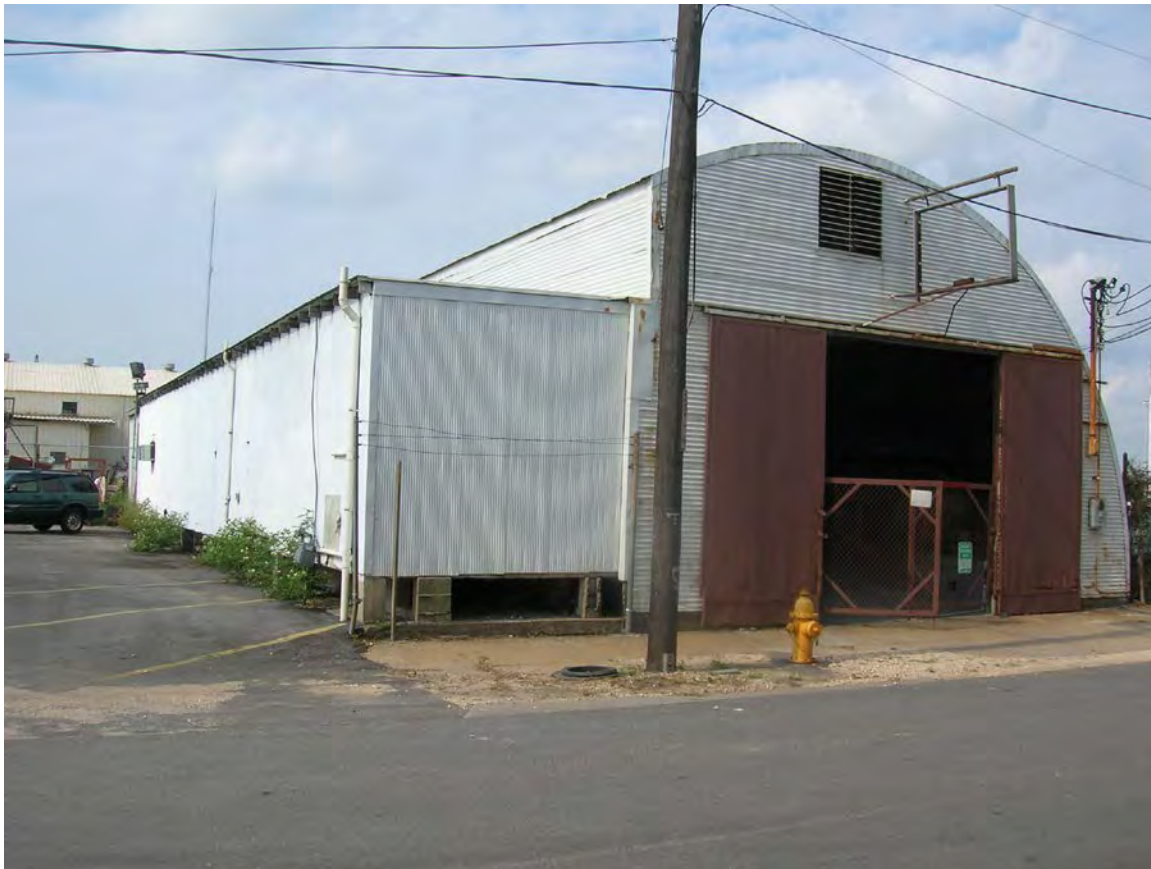
Figure 43. View to the southwest of the front of former Bender Structure 1, Electrical Maintenance Shop, on Eslava Street.
