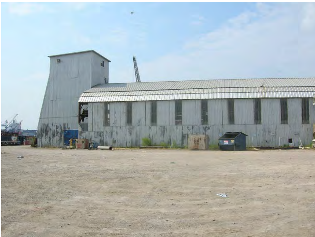
Figure 22. Closed workshop for Testing and Training Department attached to Structure 3, Hull Fabrication Shop. View to the south.
