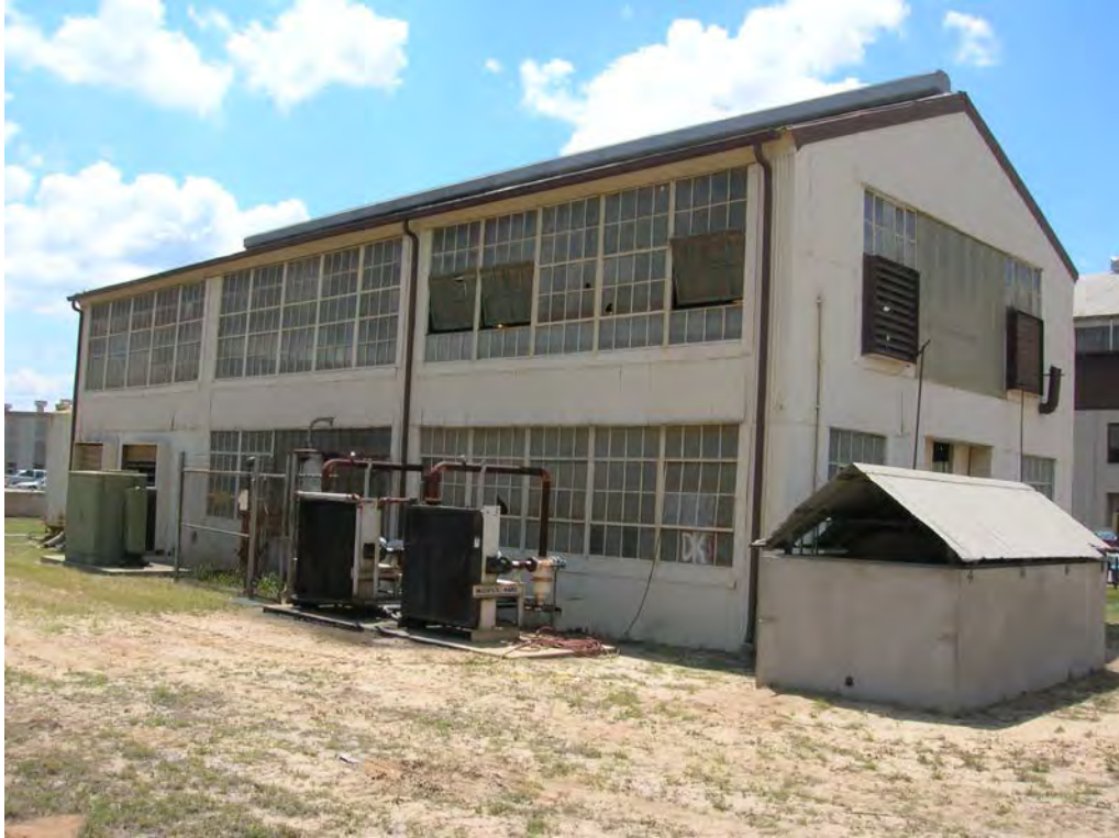
Figure 15. South side of Structure 3, originally tool house, currently pump house. View to the southeast.
