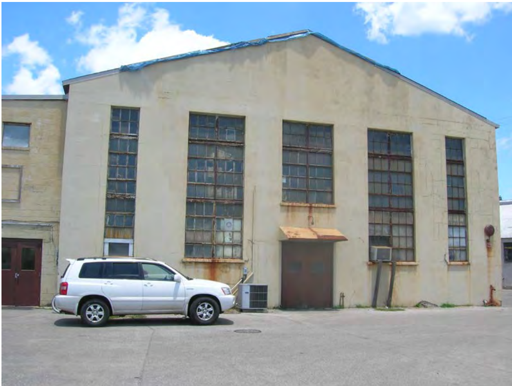
Figure 27. Front of Structure 8 Maintenance Building at BAE Systems Southeast Shipyards. View to the north toward Alternates A, B, B’, and C.
