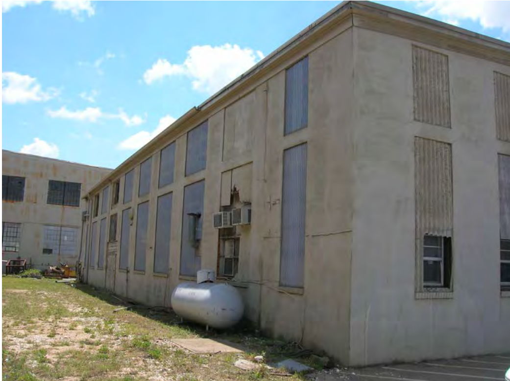
Figure 19. North side and front of Structure 4, electrical shop. View to the southeast.
