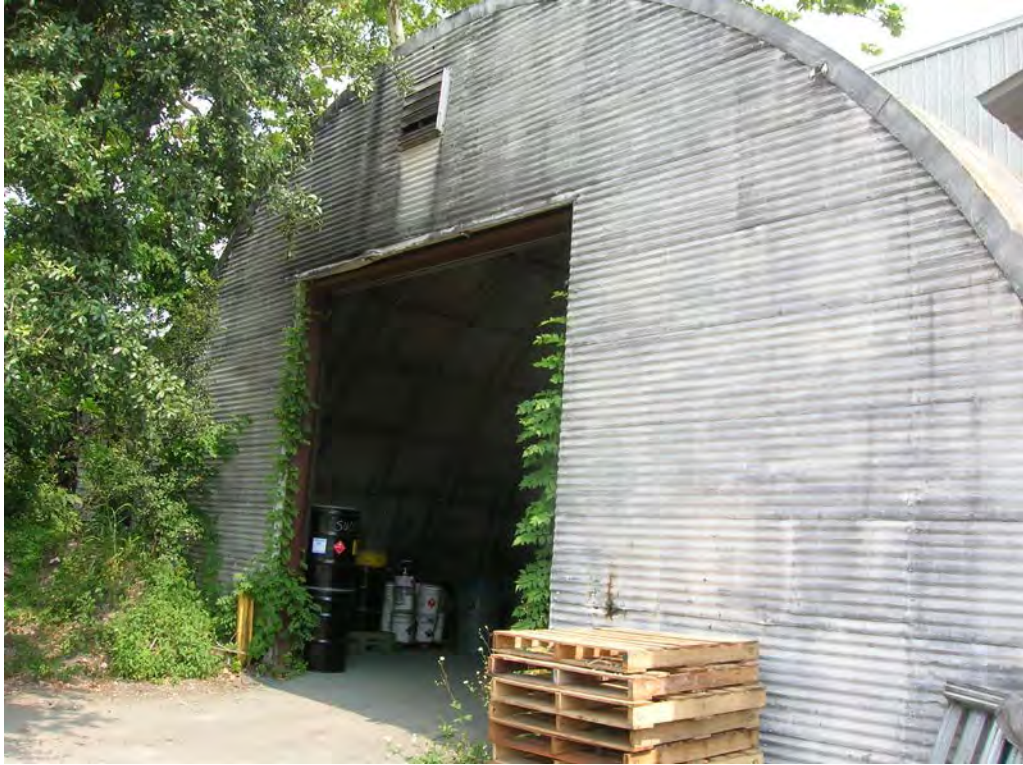
Figure 33. Front of Structure 5, Quonset hut, originally Radcliff Gravel Company, former Bender Paint Kitchen. View to the northwest toward Alternates A, B, and B'.
