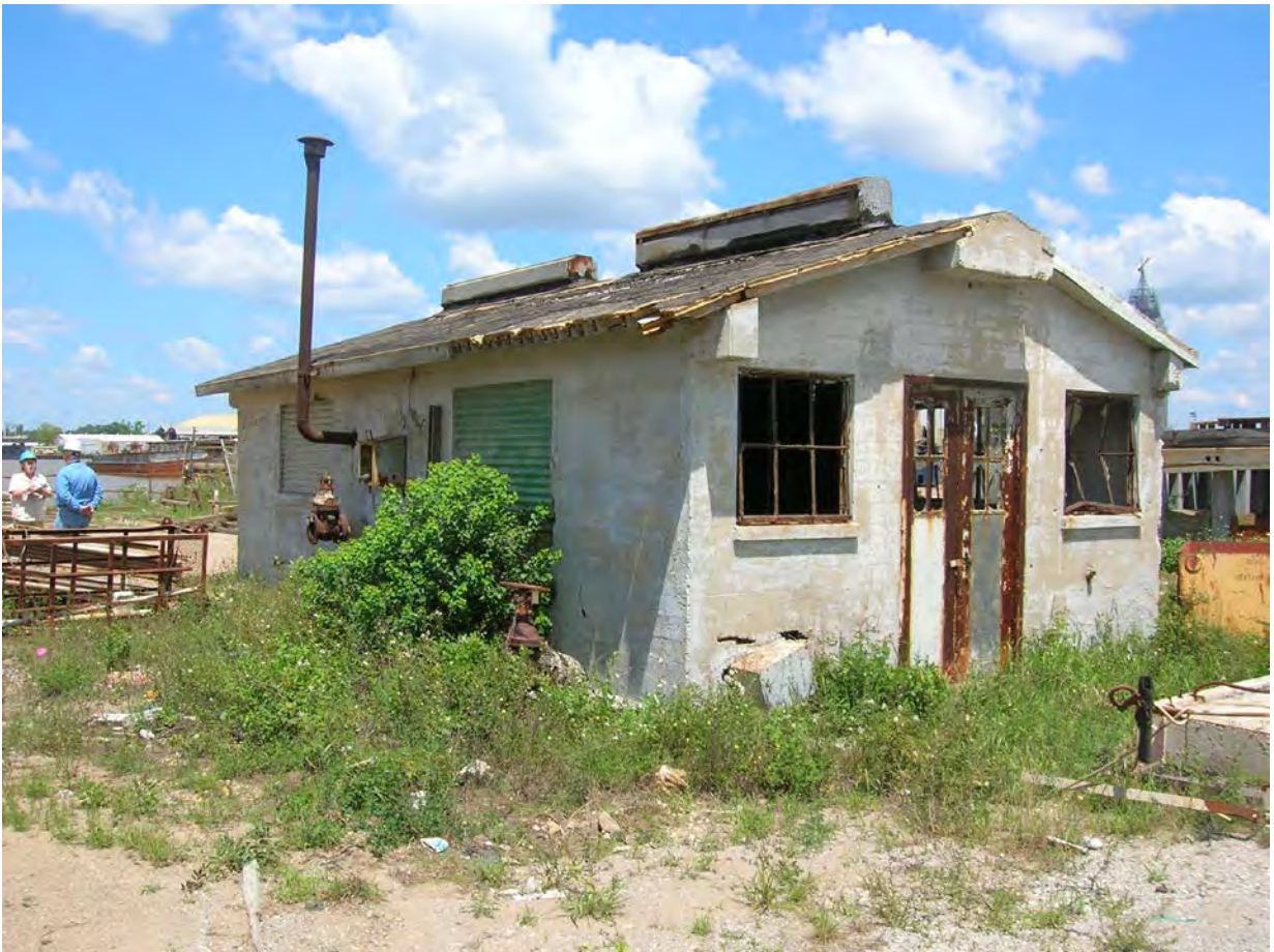
Figure 13. Structure 2, Pump House at BAE Systems Southeast Shipyards. View to the northwest toward Alternate C.
