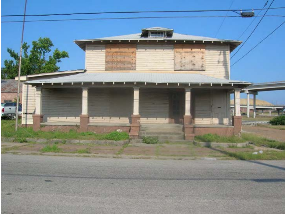
Figure 50-1. View to the west of “Union Hall” (Resource 50), originally built as a residence and later used by a shipyard worker organization, on S. Royal Street.
