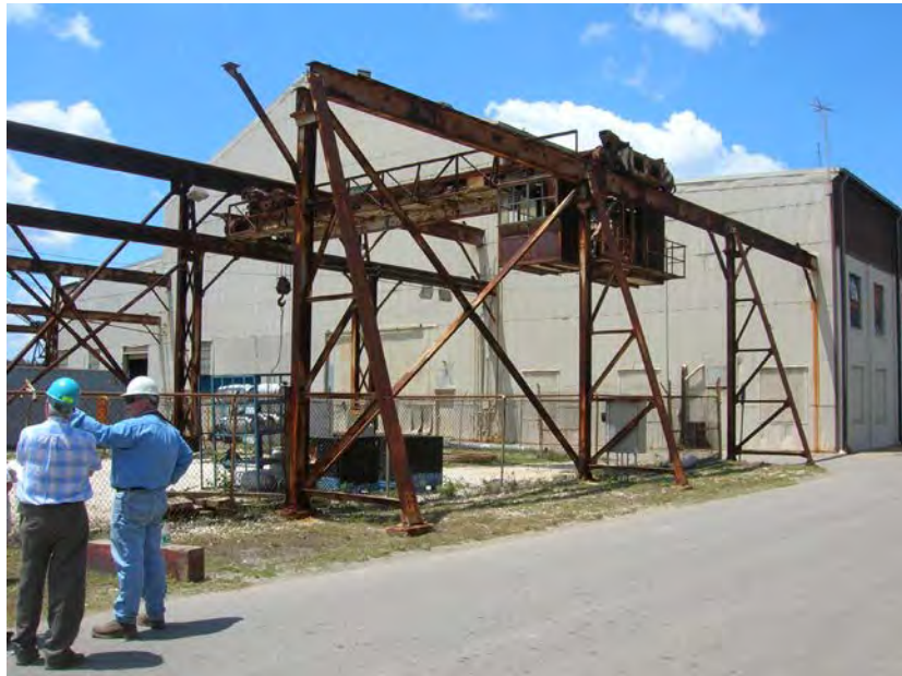
Figure 31. Overhead cranoes at the rear of Structure 10, originally machine shop, currently services buildings at BAE Systems Southeast Shipyards. View to the southwest.
