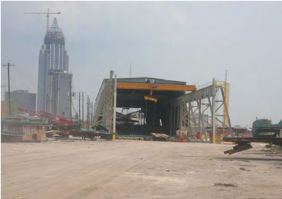
Figure 35. South end of Structure 6, Panel Line Shop at the former Bender Shipyard. View to the north toward Alternates A, B, and B'.
