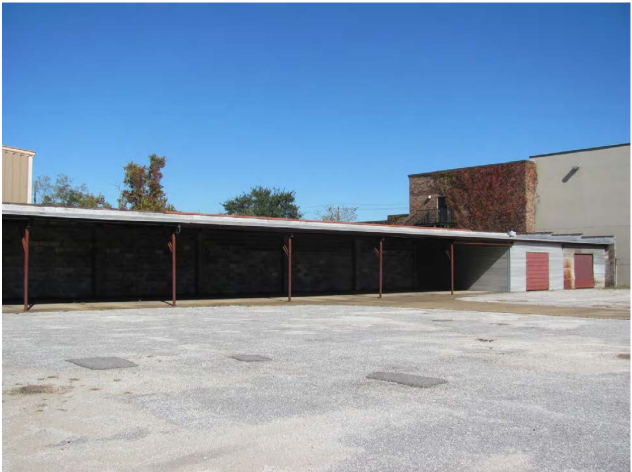
Figure 33. View to the northeast of Structure 19c, metal open bay parking garage for A.W. Williams Inspection Co., Inc. on Survey Block 32.
