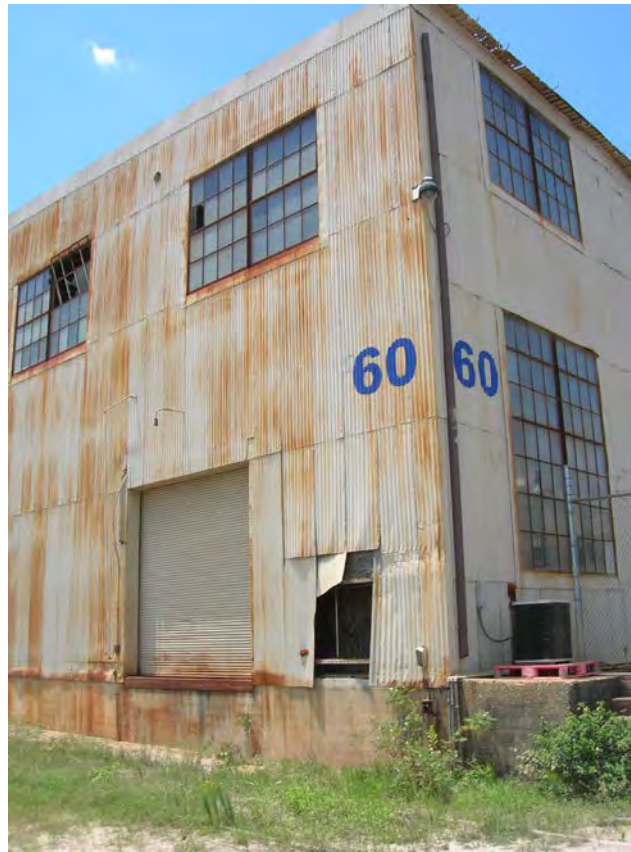
Figure 36. Structure 12, Warehouse No. 3 at BAE Systems Southeast Shipyards. View to the southeast.
