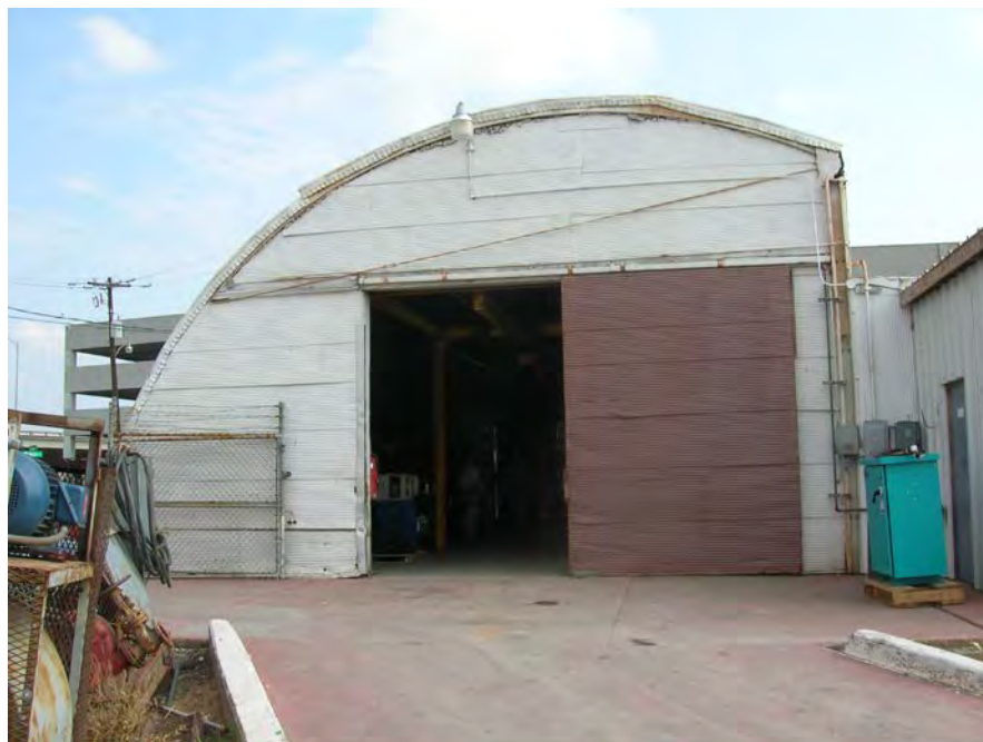
Figure 16. Rear of Structure 1, electrical maintenance shop, showing the cut-off east side and addition (right). View to the north toward Alternate A.
