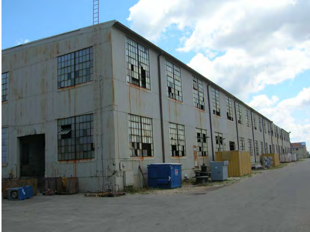
Figure 21. Front and south side of Structure 5, Warehouse No. 2. View to the northeast.
