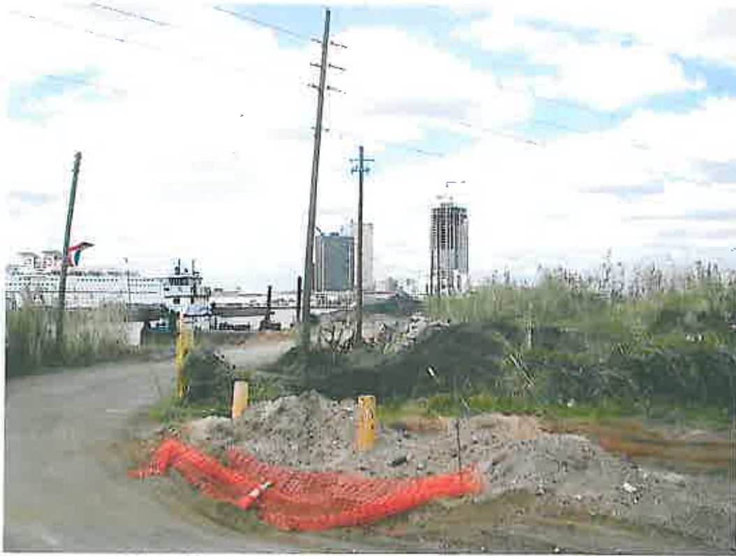
Mobile Abrasives Site looking west toward Mobile River. (Alternatives B and B')
